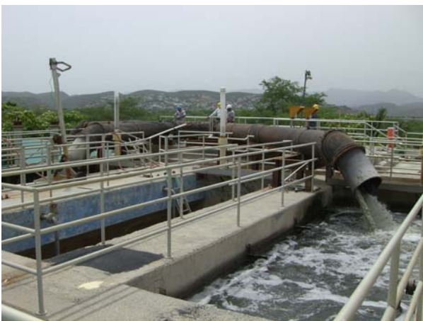
Wastewater Treatment Plant
